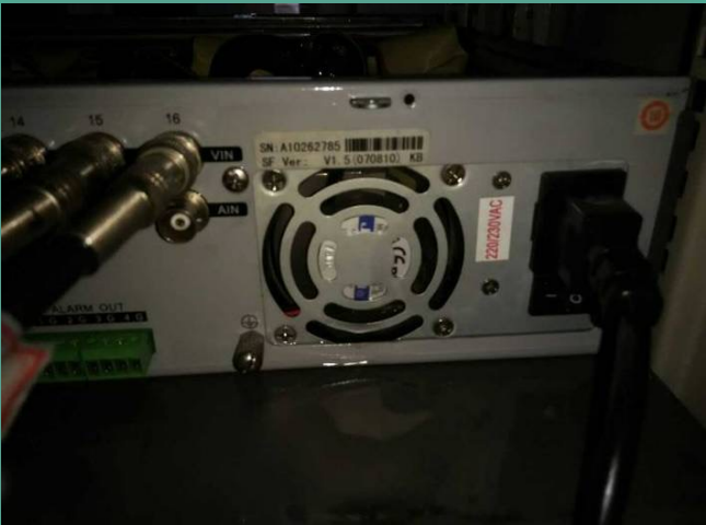
Monitoring Equipment A Data Center in Shanghai
