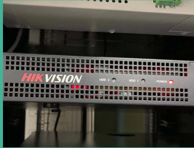
Monitoring system PetroChina Gas Station
