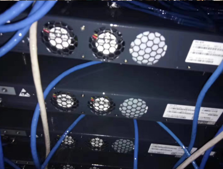
Cabinet Fans Communication Base Station A Branch of China Unicom
