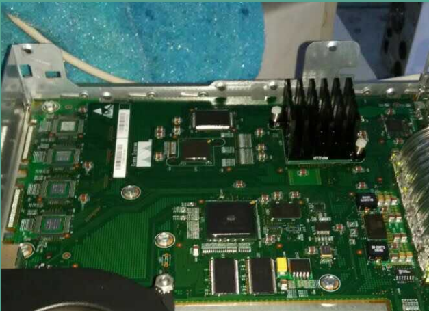
Switching Equipment Motherboard A Data Center in Shanghai
